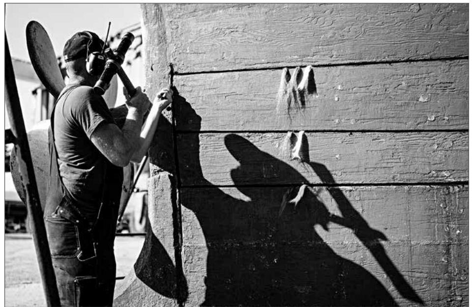
Port Townsend Shipwrights Coop - Brad Seamans uses a corking mallet and irons to wedge cotton, and then oakum into the seams in-between the planks of the fishing vessel Vansee. The boat, built in 1913, is on a regular maintenance schedule at the Shipwrights Coop to caulk three seams a year as well as any other touch-up work.
