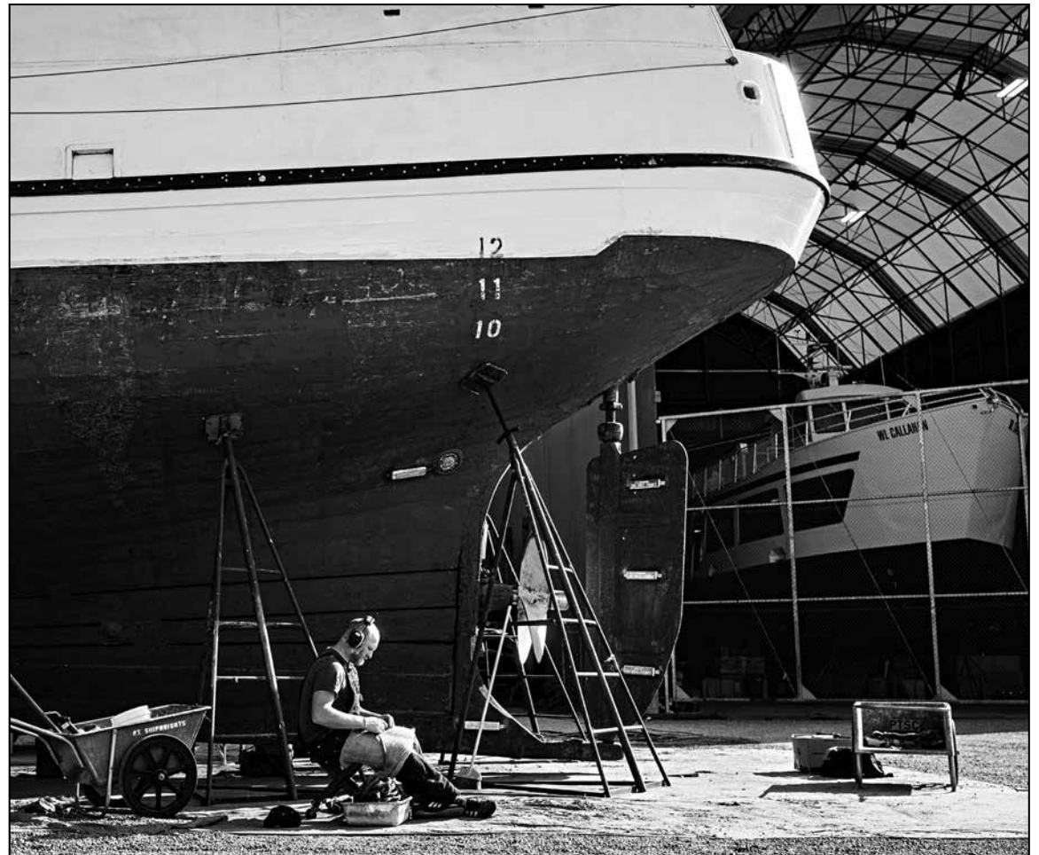
Port Townsend Shipwrights Coop - Brad Seamans, co-owner and shipwright, spins oakum under the hull of the fishing vessel Vansee, a Halibut Schooner built in 1913. The Vansee is one of four similar boats that the Shipwrights Coop has started working on after the closure of the Fishing Vessels Owners boat shop in Seattle.
